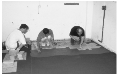
Figure 8.16e — Vibrated floor process — epoxy slurry bond coat is troweled onto fresh screed. Porcelain pavers are installed into the fresh epoxy slurry bond coat.
