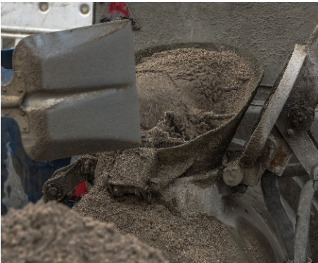
Figure 8.16a — Vibrated floor process — Mortar is mixed and pumped to area in a combination mortar mixer/pump combination.
