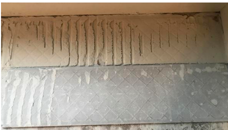
Figure 8.6 – Example of incomplete bedding due to lack of sufficient mortar and/or incorrect trowel size selection and beat-in.
