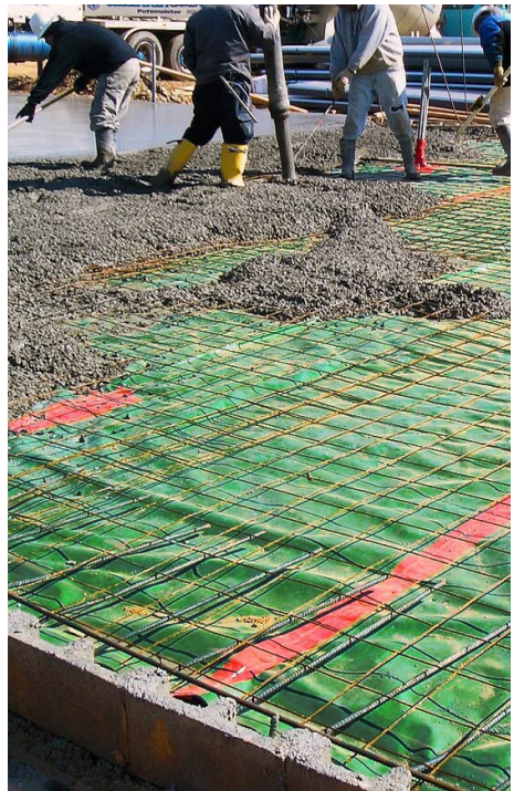
Figure 2.13 – Placement of vapor retarder over blatter layer / directly under the concrete pour.
