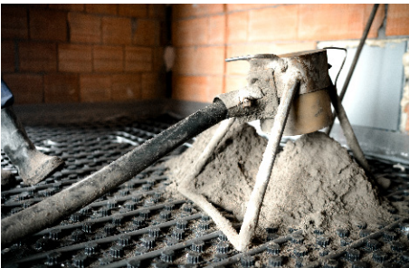
Figure 8.16b — Vibrated floor process — screed mortar is discharged onto floor area from the mortar pump.
