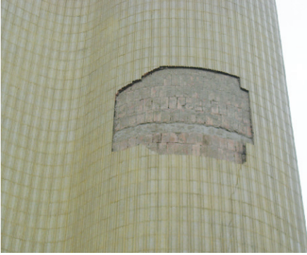
Figure 5.2 — Result of improper tile selection for the application. The use of a semi-vitreous tile — 7% in absorption did not stand up to the demands of this installation.
