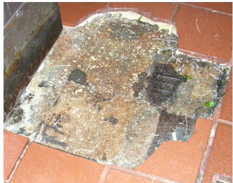
Figure 7.9 – Effects of inappropriate grout used on an industrial application. Notice not only the erosion of the grout joints, but also the adhesive mortar under the tile. In most industrial floor applications, the use of an epoxy-based adhesive and an industrial epoxy grout are required in order to ensure long-term performance.
