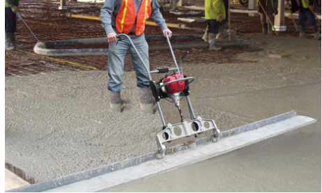
Figure 8.16c — Vibrated floor process — mortar is screeded with a vibrating screed to the desired height and pitched.
