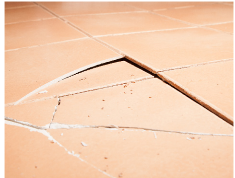
Figure 2.4 — Result of stresses induced by concrete shrinkage and lack of movement joint control. As the concrete shrinks, expansion joints are required to relieve the stress. When expansion joints are omitted or are not sufficient, “tenting” of the tiles can occur, creating bond failure and cracking.
