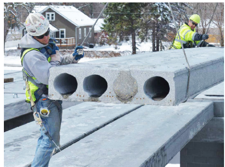
Figure 2.24 — Pre-Cast Concrete Planks. Planks rest and are supported by a flange attached to the steel girders. The planks are hoisted into place by a crane and mortared to the beams and to each other. Photo courtesy of Country Materials Corporation. 16
