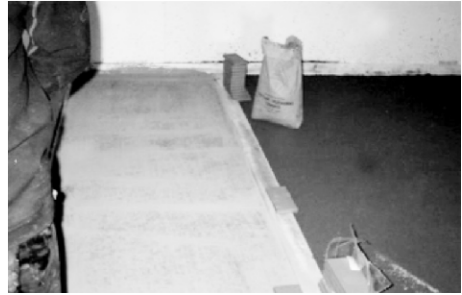
Figure 8.16d — Vibrated floor process — floor is squared and prepared to receive quarry tile floor.
