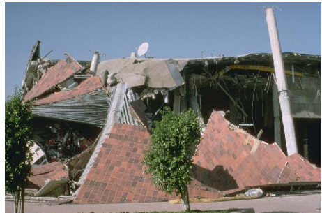
Figure 7.2 — High adhesive shear and tensile strength to resist seismic movement. Photograph of the Bullocks building after the Northridge California earthquake in 1994. Tiles remain adhered after severe shear stress from seismic activity and structural failure.
