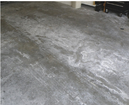
Figure 2.19 — Presence of Efflorescence on surface of concrete slab. Moisture migration through the slab can carry destructive salts to the surface of the concrete slab.
